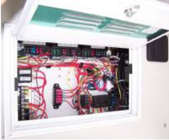
Fig. 7 - Power Distribution Center
