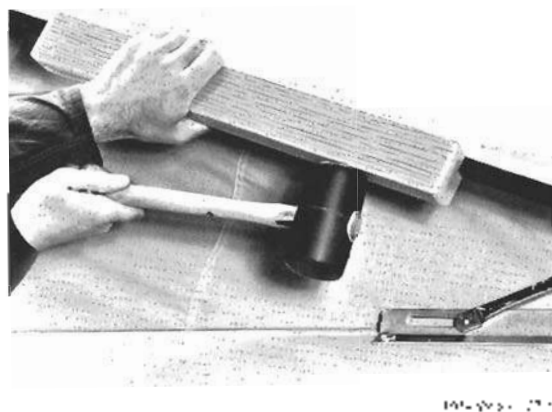
Fig. 7-36. A wooden block and rubber mallet being used to drive the seal fully into place.
