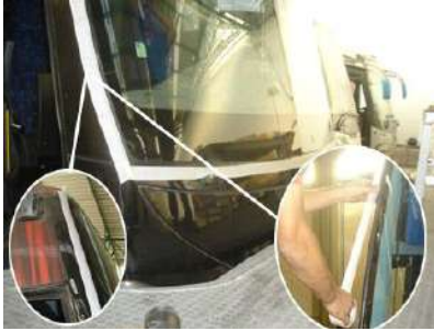
Masking tape surrounding the windscreen hole
