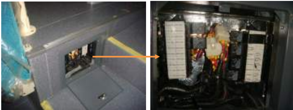
The relay and fuse box (detailed definition could be found on Wiring Harness)
