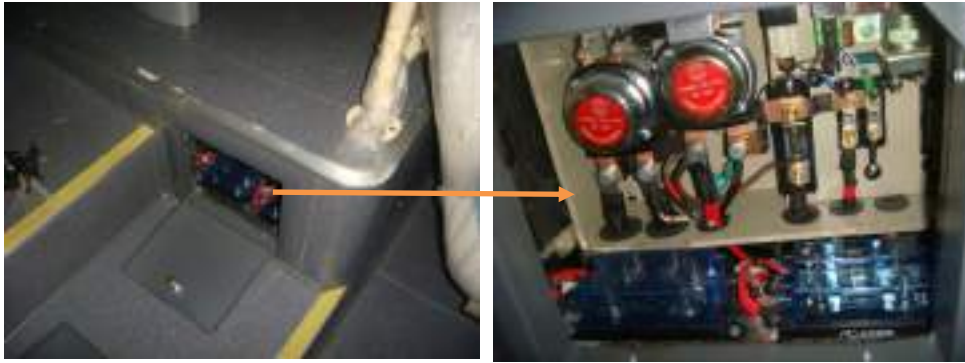
The position of switch control box
